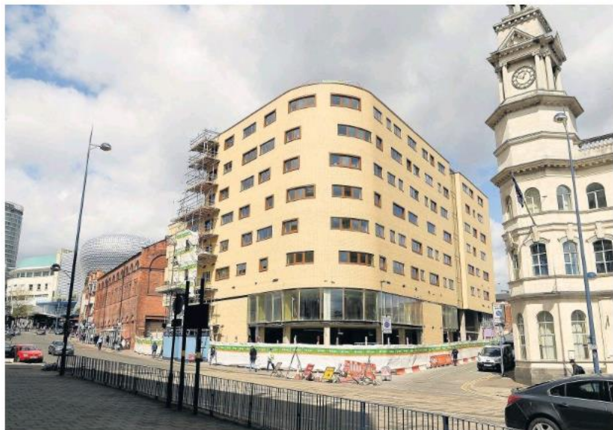
> The 110-bedroom Adagio Hotel on the corner of Allison Street and Digbeth High Street forms the first part of the Beorma Quarter in Eastside
